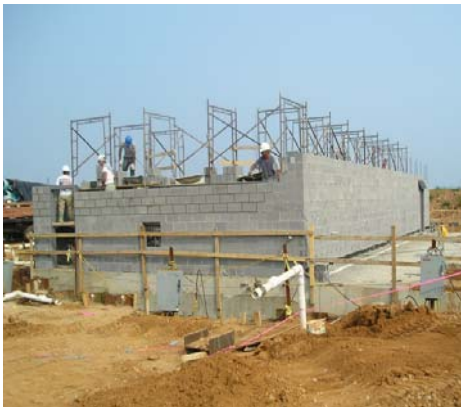
National Harbor, Wastewater Pumping Station
